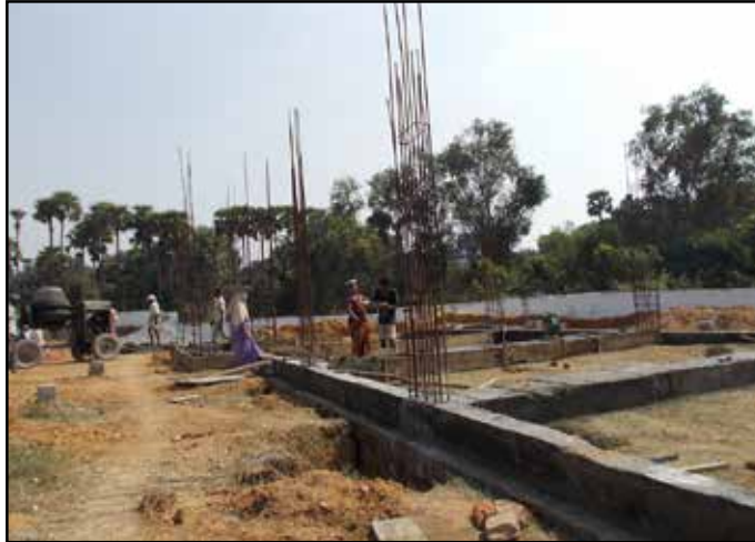
Clockwise from top: The progress on the chapel foundation; the cement mixer pulled by an autorickshaw; the men pushing the cement mixer the last 100 ft. to the work site.
