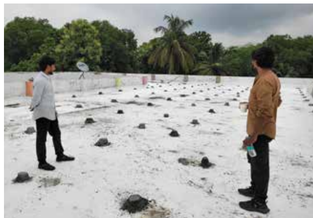
Roof contractor Kranthi and HOINA Trustee Krishna inspect the slope guides prior to pouring the final cement slab on top of the waterproof coating.
